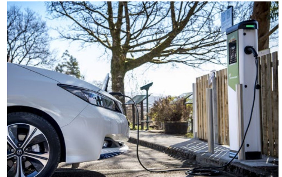
Fig. 22 - Electric vehicle charging point.
