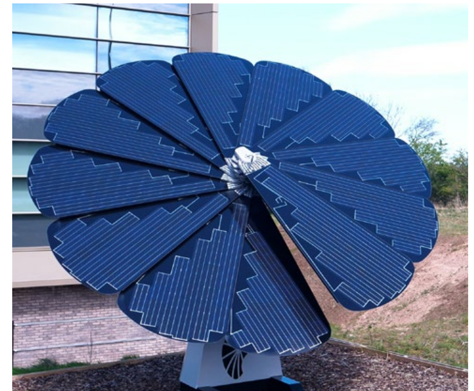
Fig. 24 - Existing solar panels installed on SEZ site.
