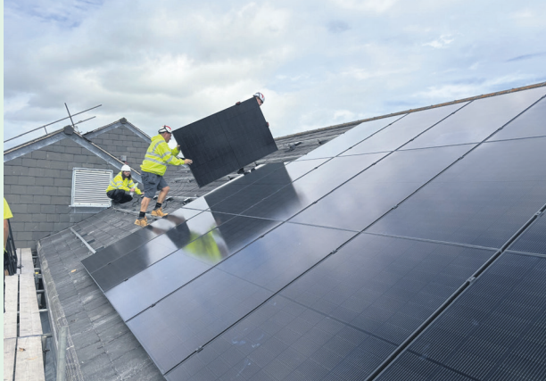
▲ POWERING UP – the panels will power the council offices with any excess going back to the National Grid.
