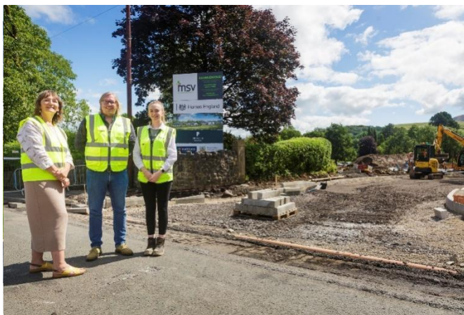
Crow Trees Brow in Chatburn, where 37 affordable properties are currently under construction.
