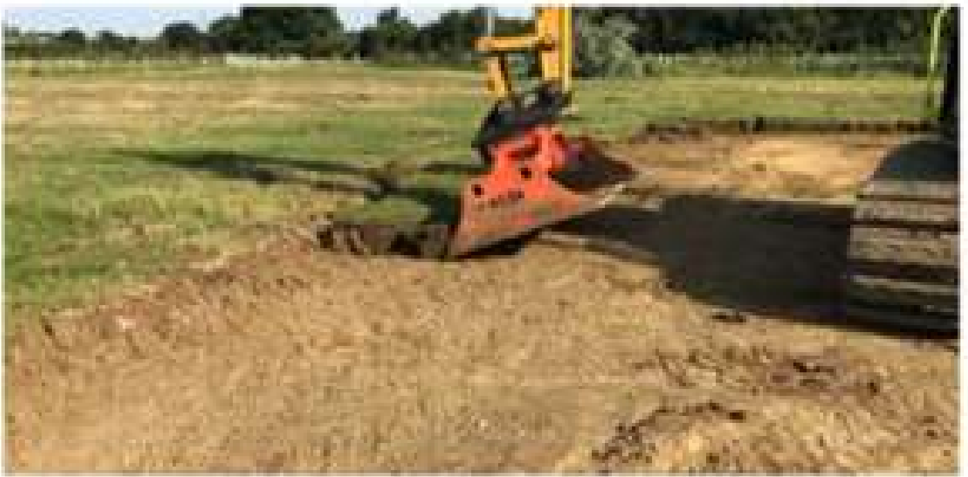
Figure 2b: Modified turf cutter used for taking turves from the trailer and placing at the receptor site.
