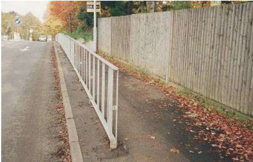
Excessive and unnecessary amounts of pedestrian guard rail should be avoided. Courtesy: David Davies.
