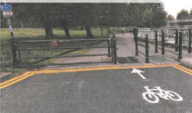
Figure 8.4: Cattle grid access control, Cambridge
