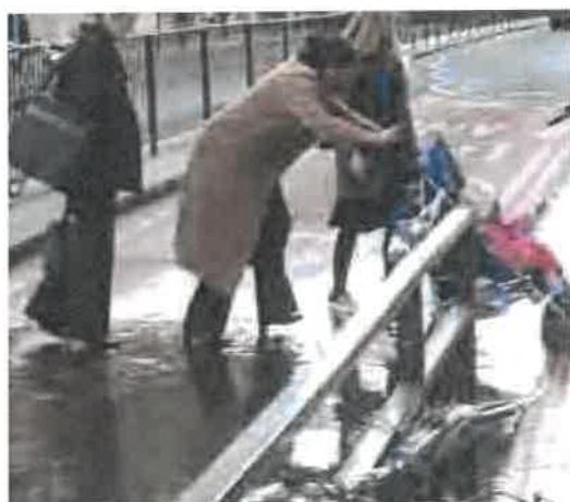
Figure 6.13 Poor drainage at a pedestrian crossing place causes discomfort and inconvenience.
